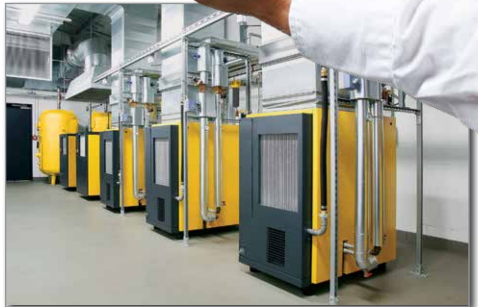
Air-cooled, fluid-injected screw compressors with internal heat exchangers and controls to tap into the thermal energy of the cooling fluid. The additional ducting removes the hot air that was not rejected by the hot water recovery system.
